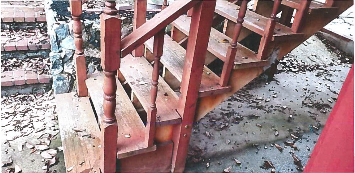
Staircase wood leading to deck is deteriorated and rotted
