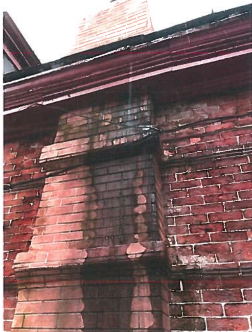
West Side chimney brick and wood trim damaged
