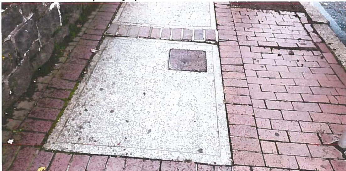
Walks are uneven and pose safety concern
