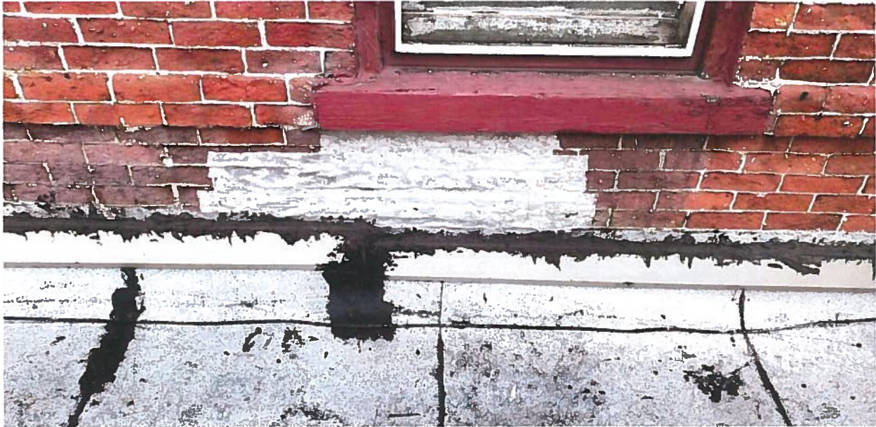
Non-professional workmanship done on side of the house
