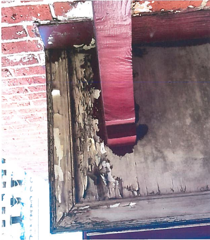
Deteriorated paint throughout
