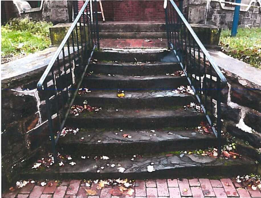
Uneven and damaged staircase in front of the house
